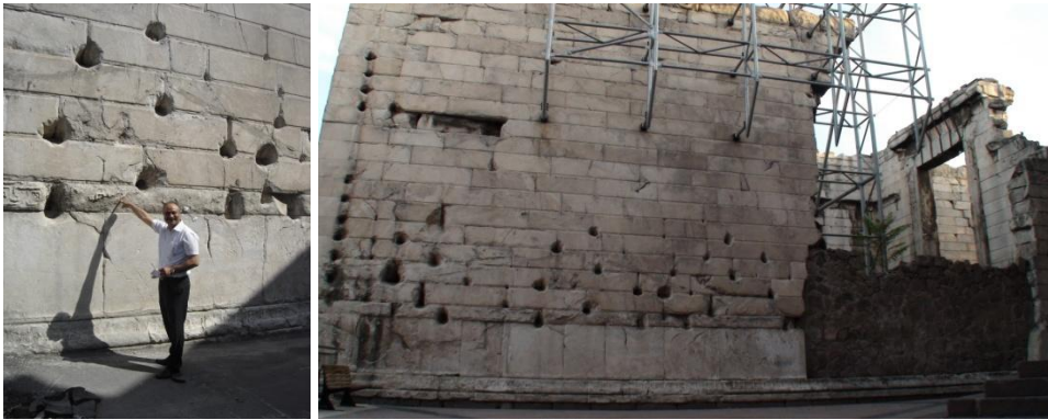
Fig 9. Deteriorations and Wrecks on the northern side walls
