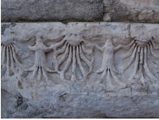
Fig 7. Deteriorations (External Walls)
