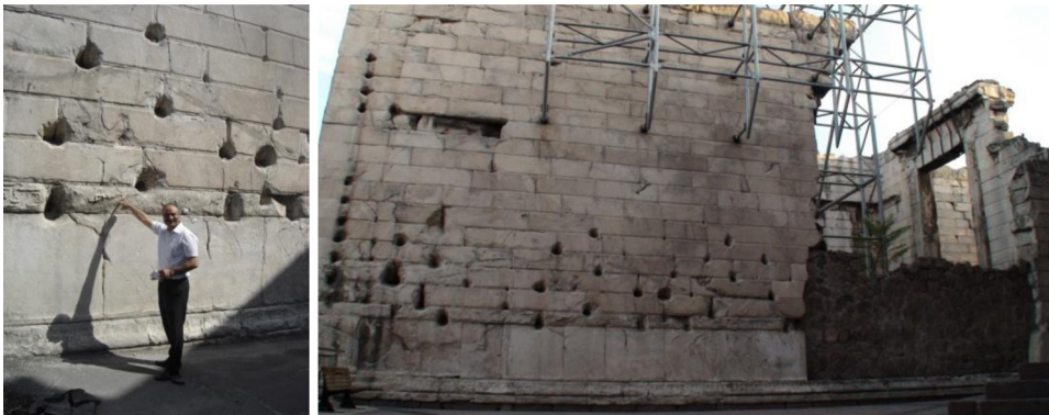
Fig. 9. Deteriorations and Wrecks on the northern side walls.
